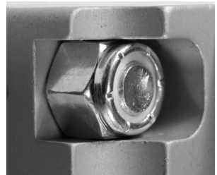
Fig 21 Bolt protrudes just beyond flush
